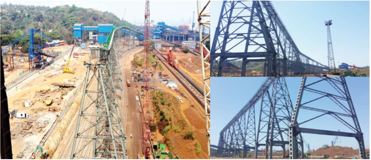
PIPE CONVEYOR SYSTEM FOR IMWLS AT SWPL- GOA
