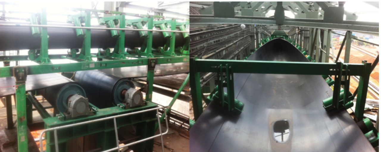
PIPE CONVEYOR AT- SOUTH WEST PORT LTD. GOA
