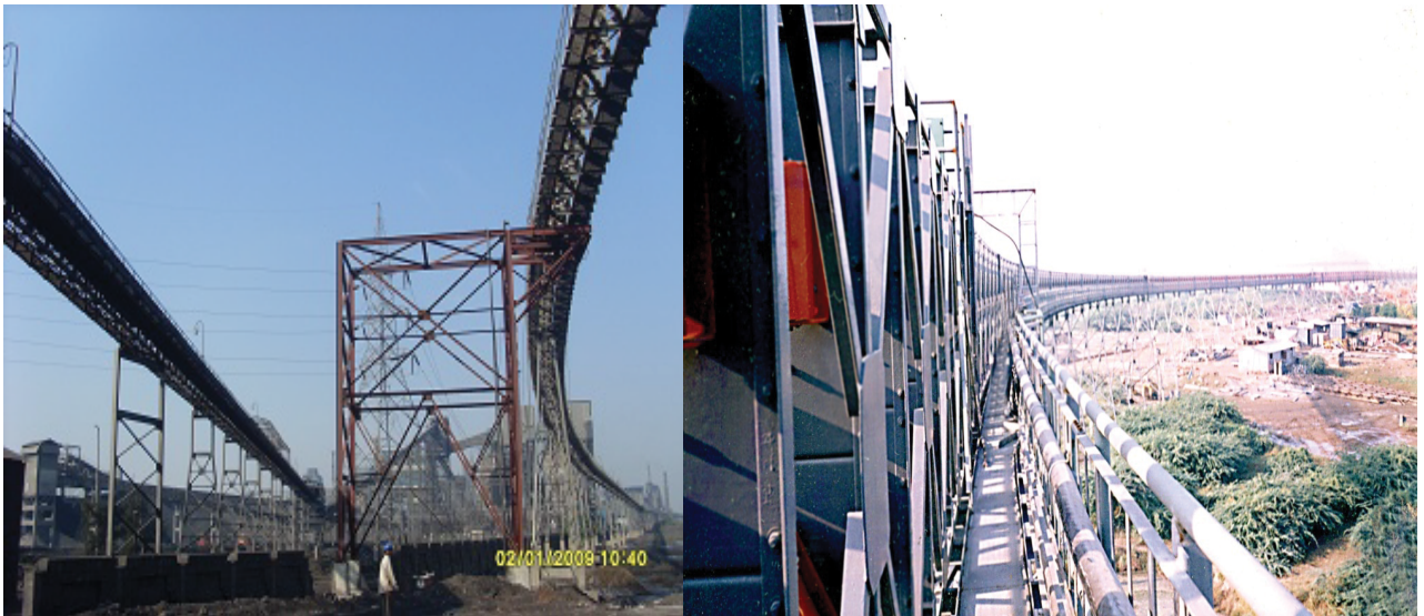
PIPE CONVEYER AT BIRLA COPPER
